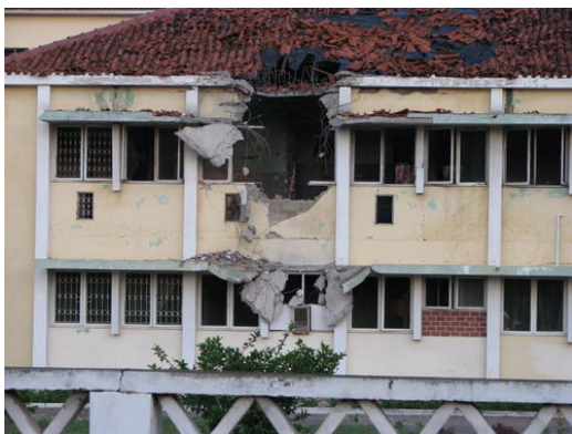
Above picture shows the damage to the Psychiatric Hospital near to the Centre.
